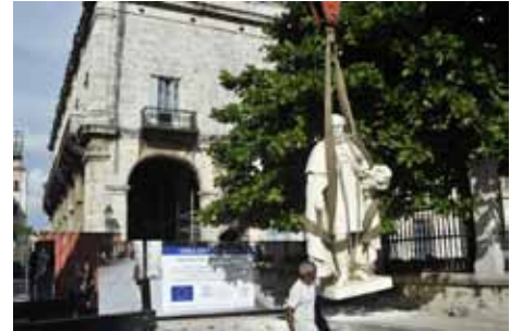
© Office of the Historian of Havana – the statue of King Ferdinand VII is transferred giving room for works in progress
